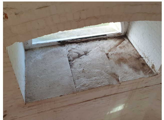
Fig 21 Staircase level windows leaking
