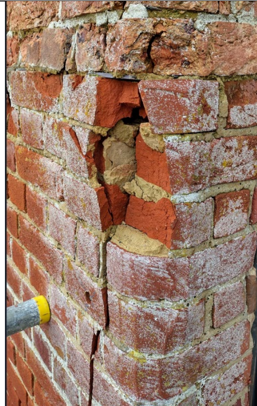
Fig 17, Significant crack at window reveal
