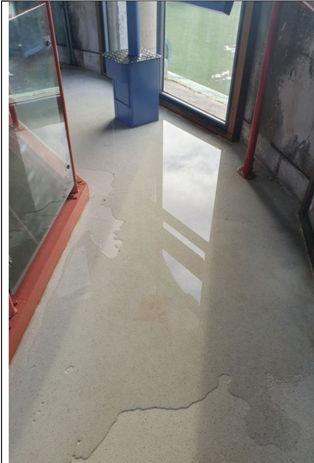
Fig 20 Upper floor windows leaking
