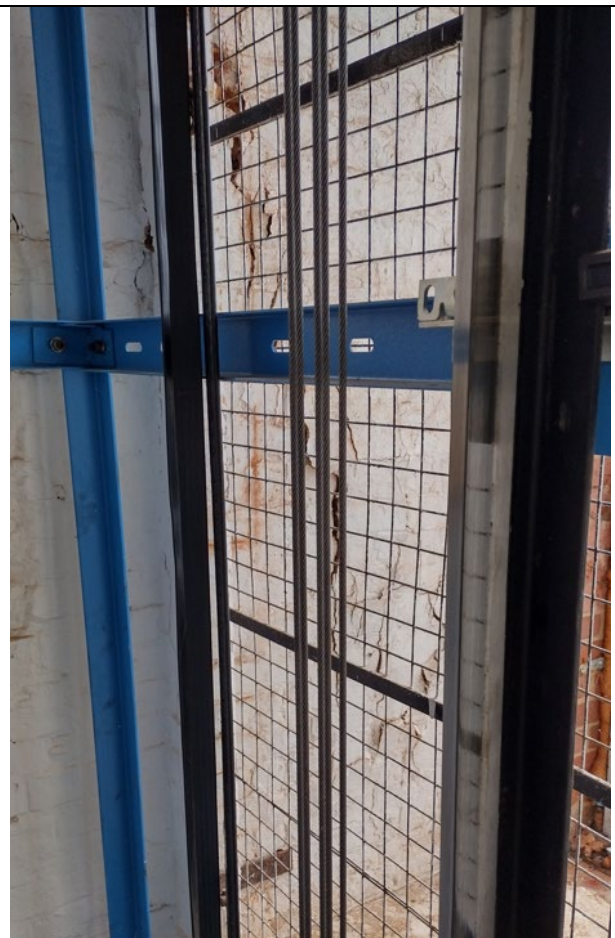
Fig 19, Lift shaft significant cracks within window reveal.
