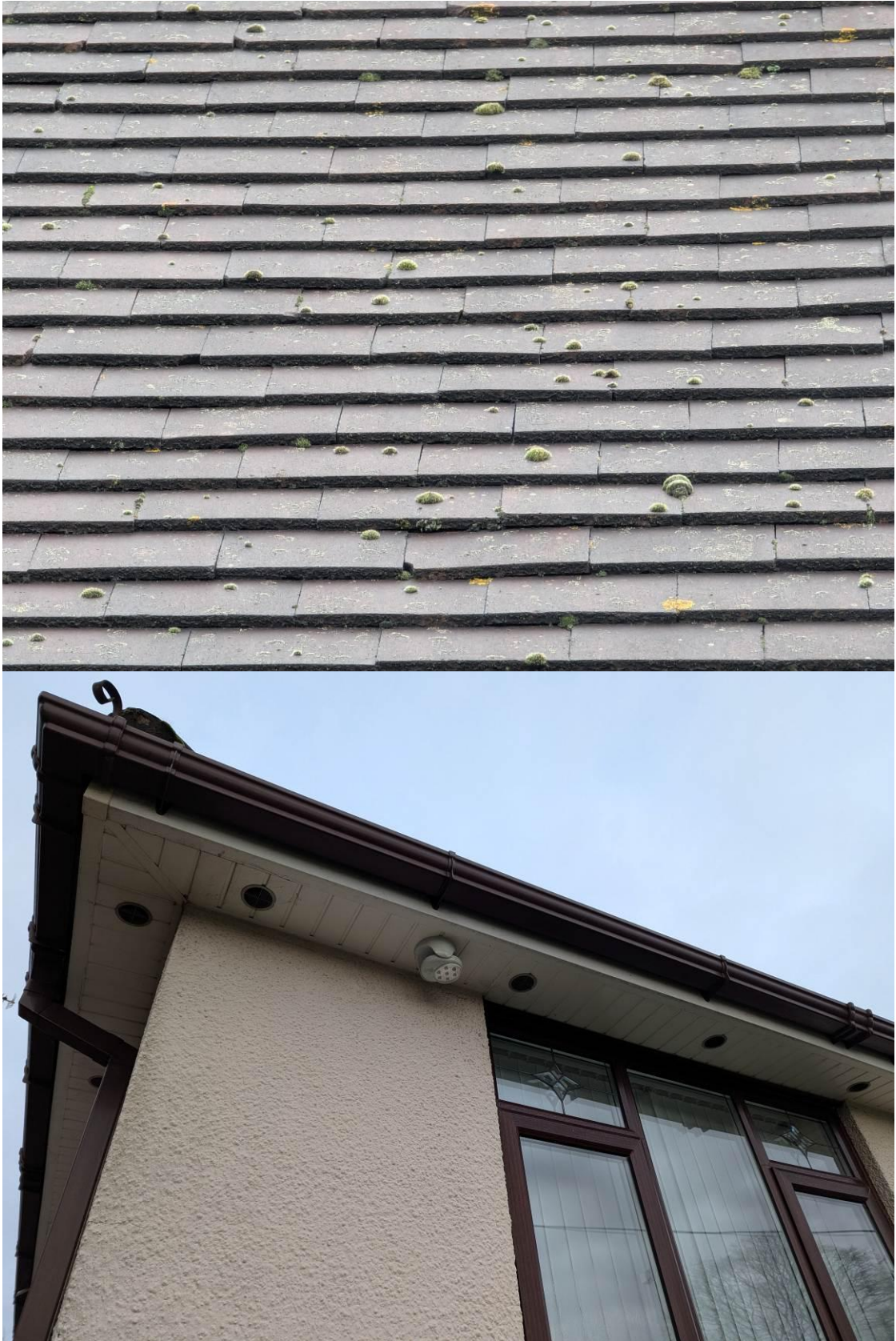
Photo 5/6 22 Trevoe Crescent Tile and soffit gaps generally very small.
