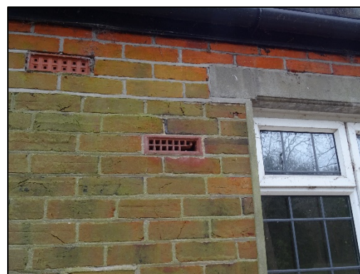
Figure 8 – damaged ventilation brick on the western elevation of the flat roof extension
