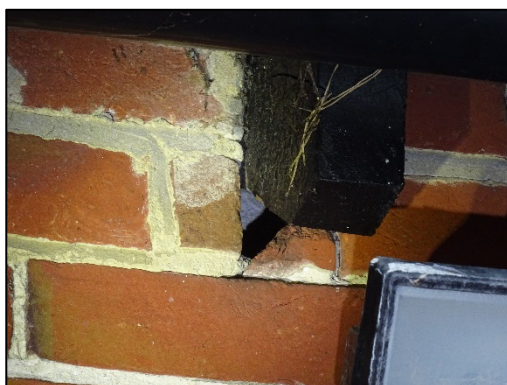
Figure 7 – hole in the brickwork underneath a beam on the southern elevation of the pitched extension
