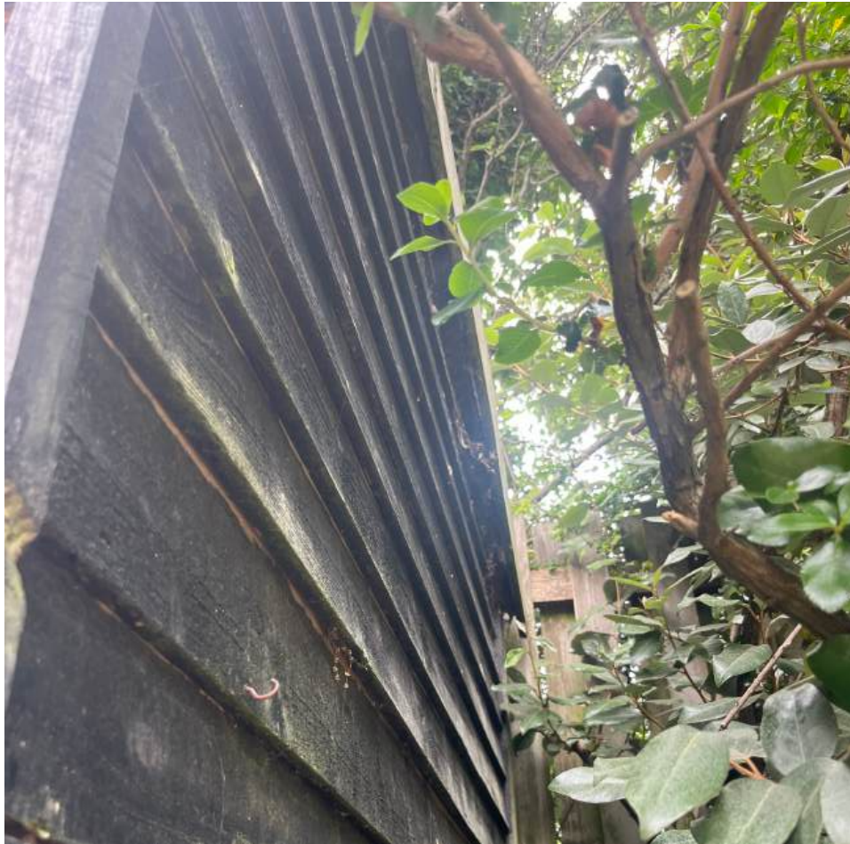
Figure 6. Close up example of the condition of the weather boarding (June, 2025).
