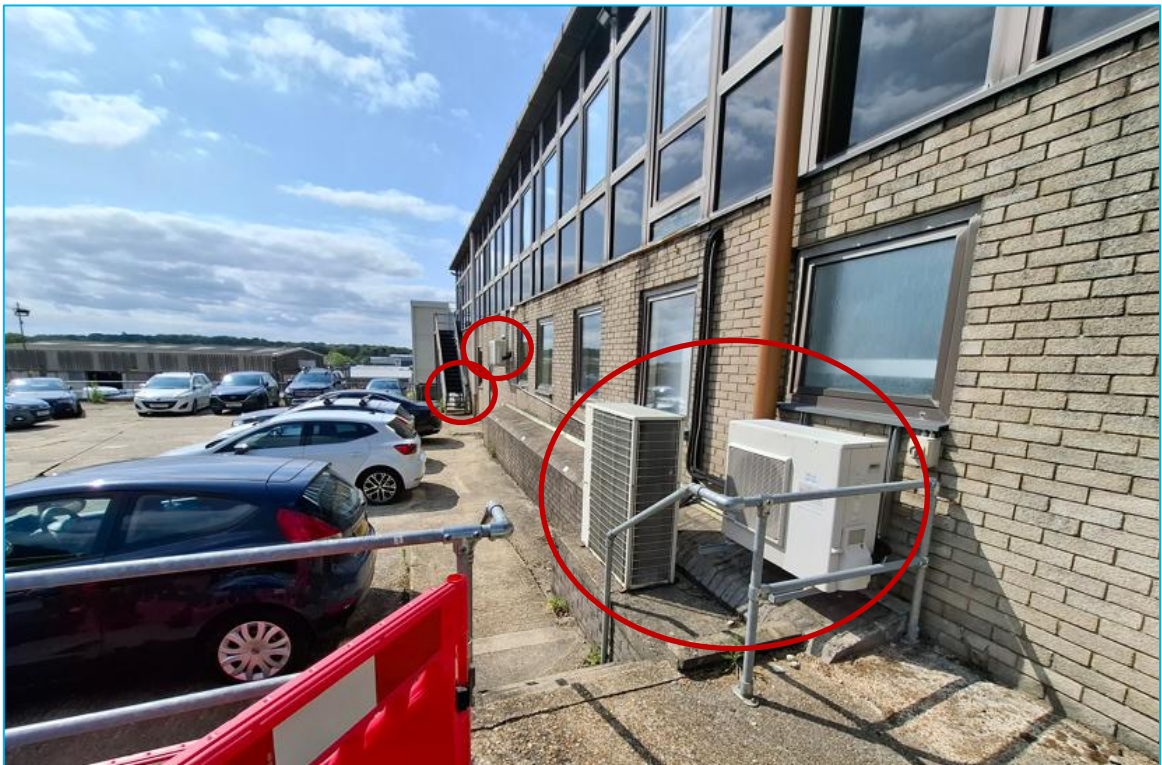
Figure 10: Existing plant on south façade (not in use at time of survey)
