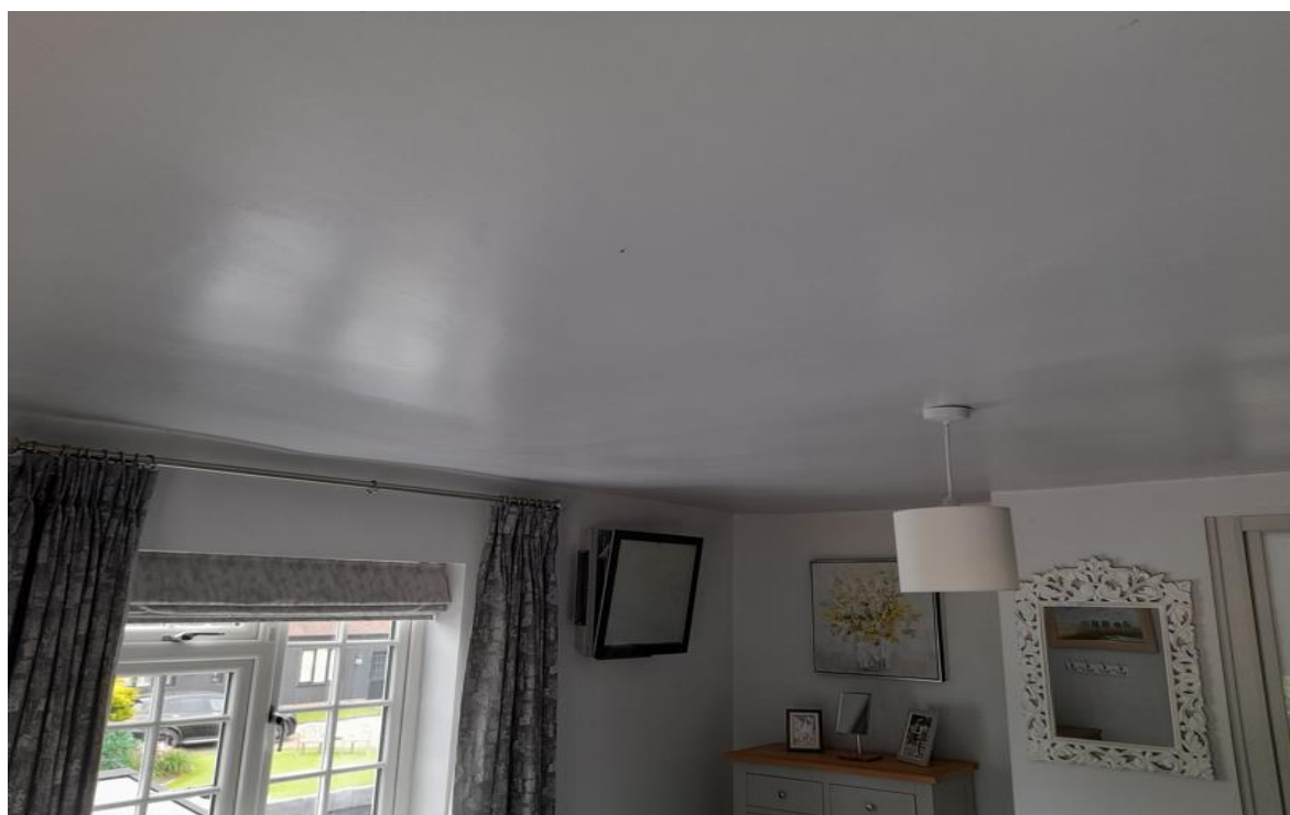
Fig. 14: Ceiling deflection in the eastern front bedroom of Stroudwood Farmhouse.
