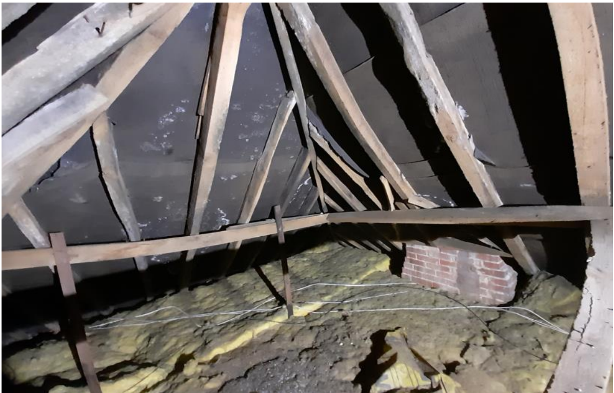
Fig. 20: Timbers at the eastern hipped end of the roof, with purlins supported on inadequate joists.
