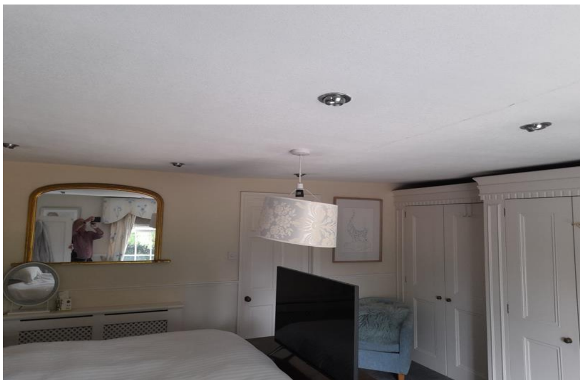
Fig. 13: Ceiling deflection in the western front bedroom of Stroudwood Farmhouse.
