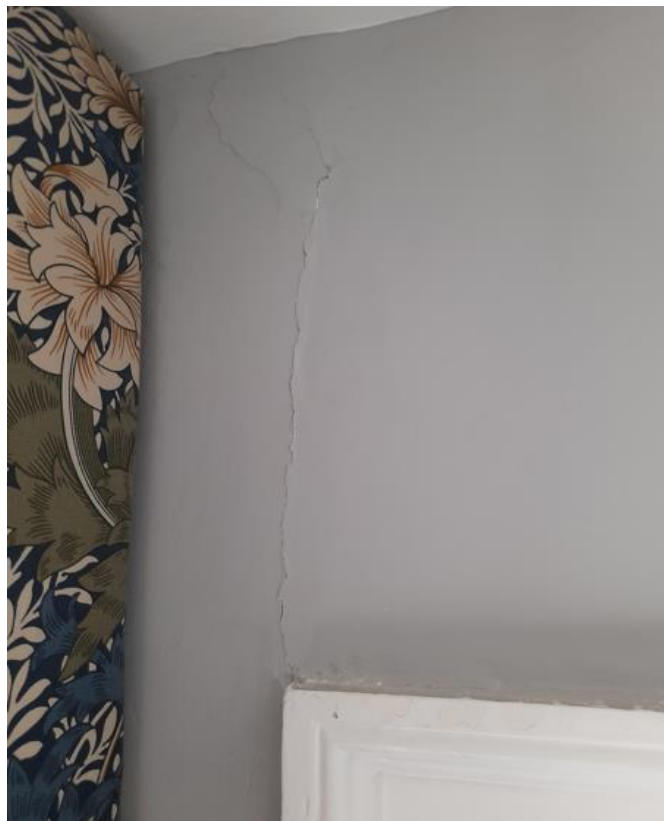
Fig. 15: Cracking in surface plasterwork on the first-floor landing.
