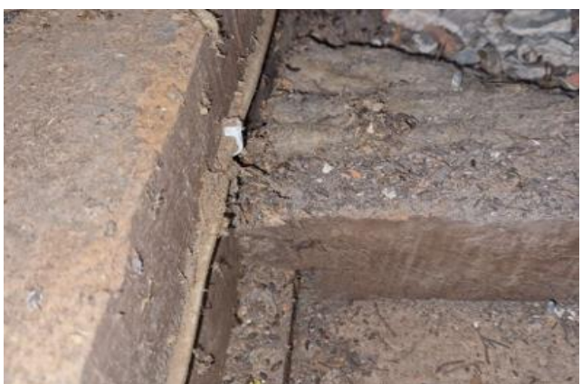
Fig. 18: A notched ceiling joist and end-bearing.
