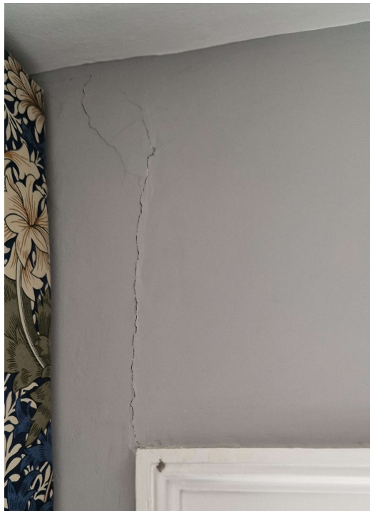
Figure 9 – Cracks above first floor bedroom doorways
