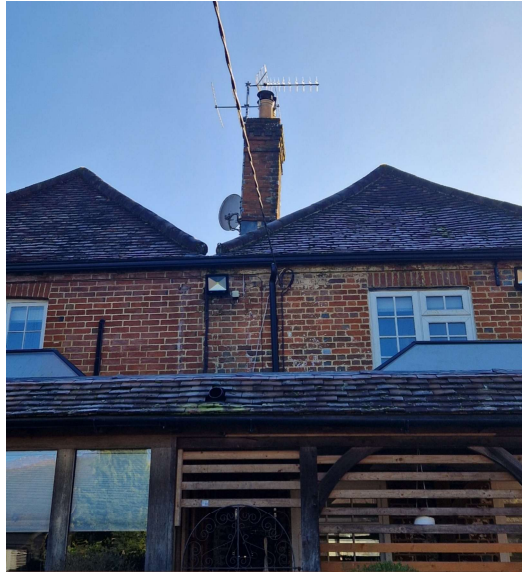
Figure 3 – Side (West) elevation of Stroudwood Farmhouse. Chimney observed to be severely out of plumb
