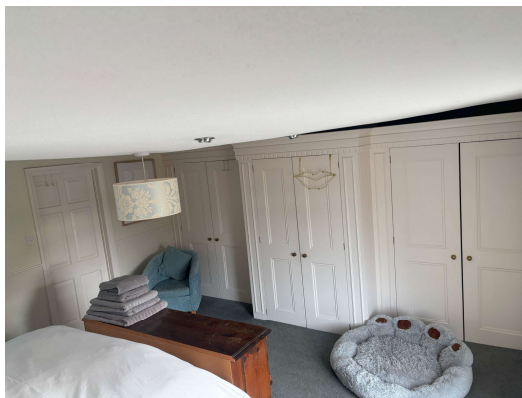
Figure 4 – Ceiling deflection of first floor bedroom
