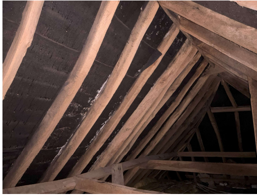
Figure 5 – Impermeable roof felt with internal condensation
