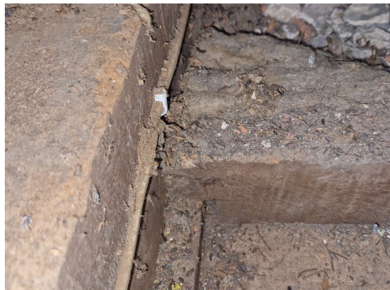
Figure 10 – Notched ceiling joists and end bearing
