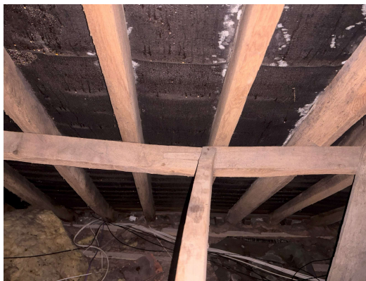
Figure 6 – Purlin joint deflecting
