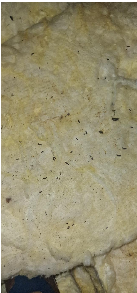
Picture 7: Showing the bat droppings on the insulation
