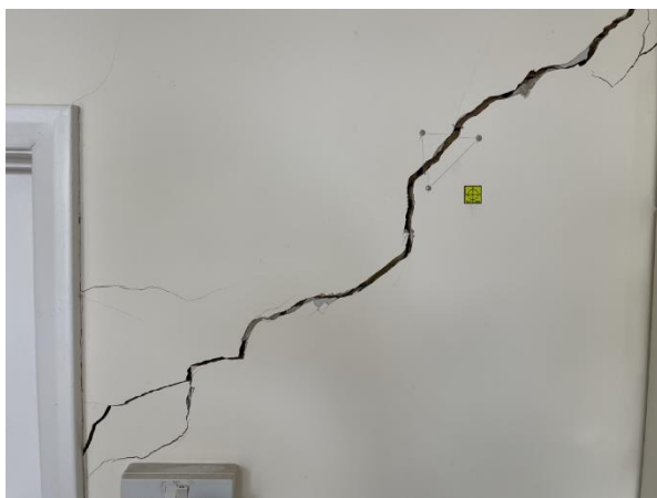
Crack between kitchen and living room (18.7.25)
