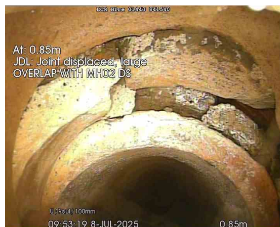
MH03 BR1_0-85m_095319.jpg, 00:00:11, 0.85 m Joint displaced, large, OVERLAP WITH MH02 DS
