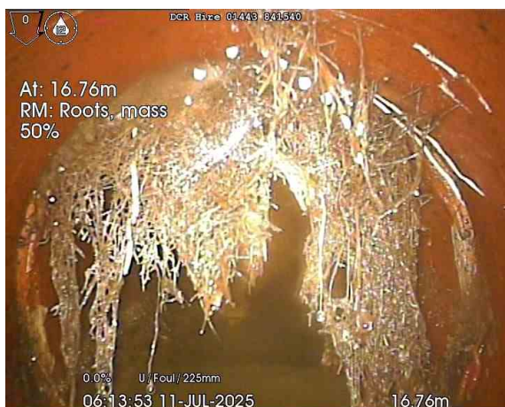
FW2301 US_16-76m_061353.jpg, 00:01:51, 16.76 m Roots, mass, 50% cross-sectional area loss
