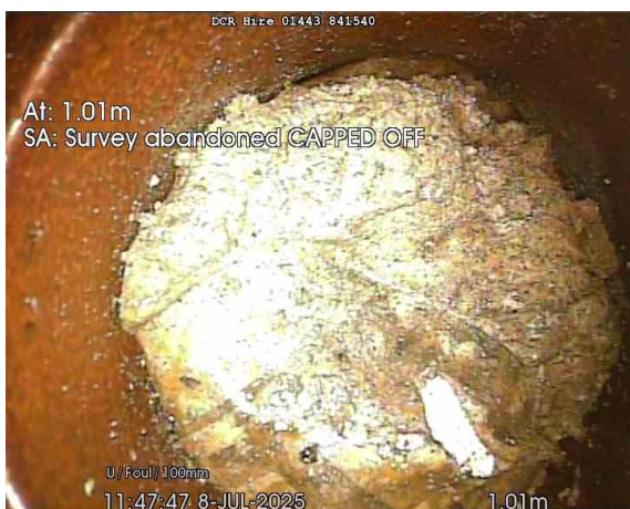
MH06 BR4_1-01m_114747.jpg, 00:00:16, 1.01 m Survey abandoned, CAPPED OFF
