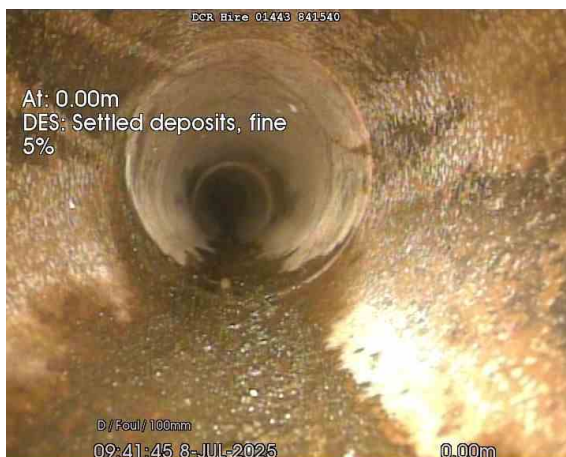
MH02 DS_0-00m_094145.jpg, 00:00:04, 0.00 m Settled deposits, fine, 5% cross-sectional area loss
