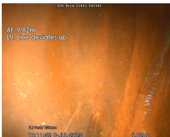
MH04 BR1_9-82m_101152.jpg, 00:00:50, 9.82 m Line deviates up
