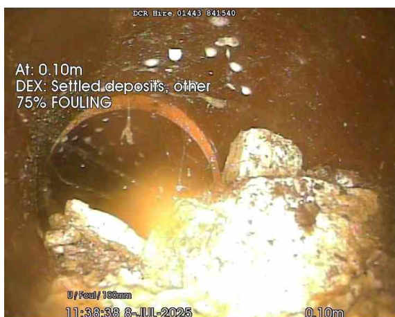
MH06 US_0-10m_113838.jpg, 00:00:06, 0.10 m Settled deposits, other, 75% cross-sectional area loss, FOULING
