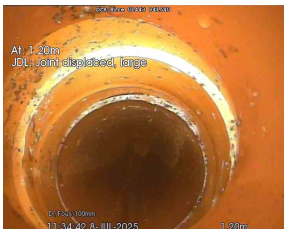
MH06 DS_1-20m_113442.jpg, 00:00:18, 1.20 m Joint displaced, large
