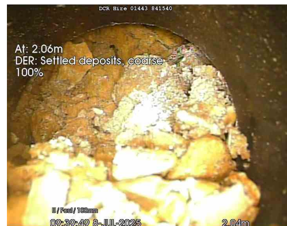
MH02 BR1_2-04m_093949.jpg, 00:00:10, 2.04 m Settled deposits, coarse, 100% cross-sectional area loss
