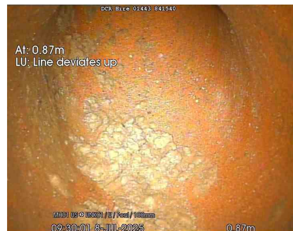
MH01 US_0-87m_093001.jpg, 00:00:12, 0.87 m Line deviates up
