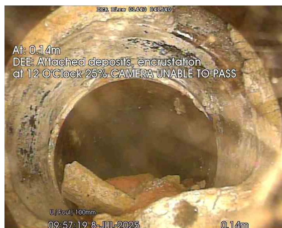
MH03 BR3_0-14m_095719.jpg, 00:00:33, 0.14 m Attached deposits, encrustation at 12 o'clock, 25% cross-sectional area loss, CAMERA UNABLE TO PASS
