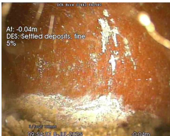
MH03 BR2_-0-04m_095437.jpg, 00:00:05, -0.04 m Settled deposits, fine, 5% cross-sectional area loss
