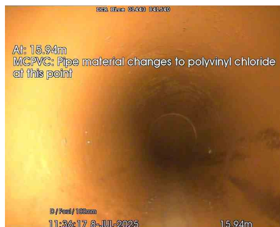
MH06 DS_15-94m_113617.jpg, 00:01:22, 15.94 m Pipe material changes to polyvinyl chloride at this point
