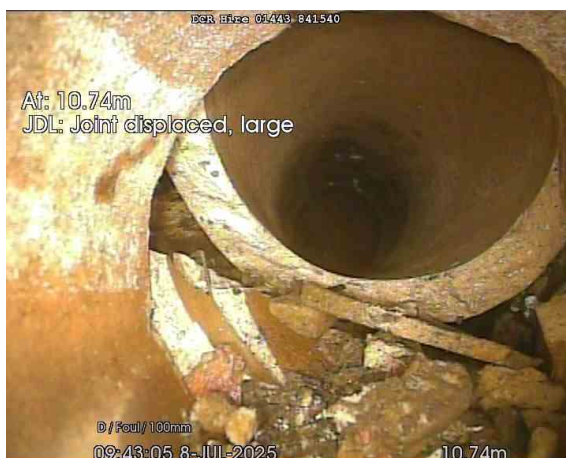
MH02 DS_10-74m_094305.jpg, 00:00:46, 10.74 m Joint displaced, large
