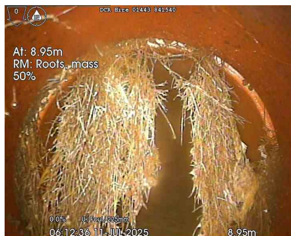
FW2301 US_8-95m_061236.jpg, 00:01:07, 8.95 m Roots, mass, 50% cross-sectional area loss
