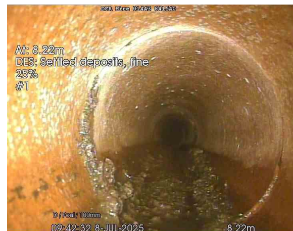
MH02 DS_8-22m_094232.jpg, 00:00:33, 8.22 m Settled deposits, fine, 25% cross-sectional area loss, start
