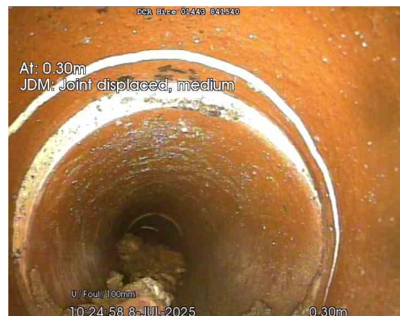
MH05 BR3_0-30m_102458.jpg, 00:00:08, 0.30 m Joint displaced, medium
