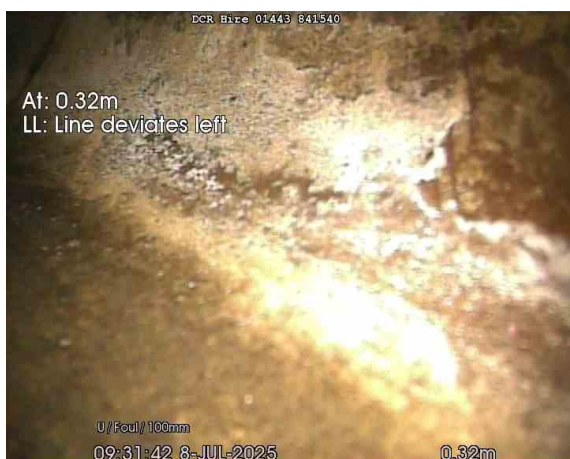
MH01 BR1_0-32m_093142.jpg, 00:00:04, 0.32 m Line deviates left
