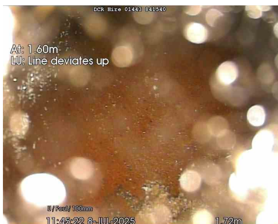
MH06 BR3_1-74m_114522.jpg, 00:00:12, 1.74 m Line deviates up
