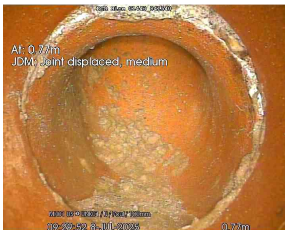
MH01 US_0-77m_092952.jpg, 00:00:10, 0.77 m Joint displaced, medium
