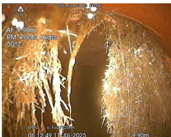
FW2301 US_9-90m_061249.jpg, 00:01:13, 9.90 m Roots, mass, 50% cross-sectional area loss
