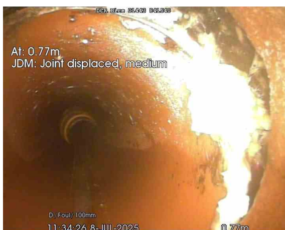
MH06 DS_0-77m_113426.jpg, 00:00:12, 0.77 m Joint displaced, medium
