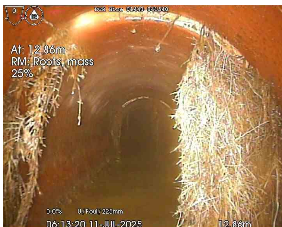
FW2301 US_12-86m_061320.jpg, 00:01:30, 12.86 m Roots, mass, 25% cross-sectional area loss
