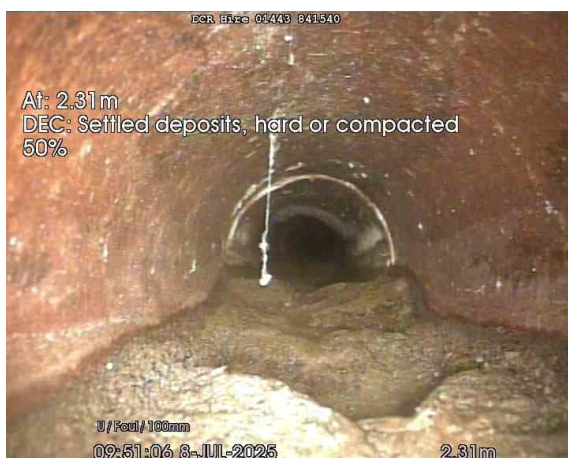
MH03 US_2-31m_095106.jpg, 00:00:47, 2.31 m Settled deposits, hard or compacted, 50% cross-sectional area loss
