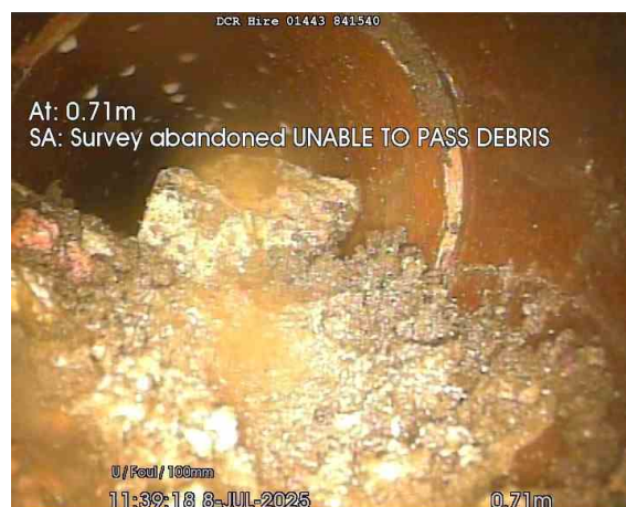
MH06 US_0-71m_113918.jpg, 00:00:16, 0.71 m Survey abandoned, UNABLE TO PASS DEBRIS
