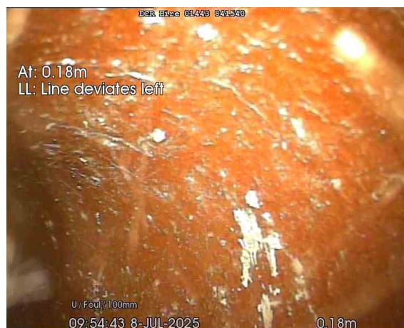
MH03 BR2_0-18m_095443.jpg, 00:00:07, 0.18 m Line deviates left
