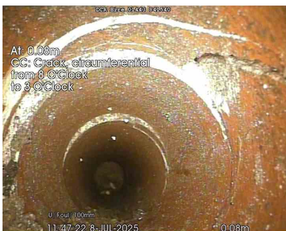
MH06 BR4_0-08m_114722.jpg, 00:00:05, 0.08 m Crack, circumferential from 8 o'clock to 3 o'clock
