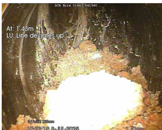
MH05 BR2_1-41m_102319.jpg, 00:00:09, 1.41 m Line deviates up
