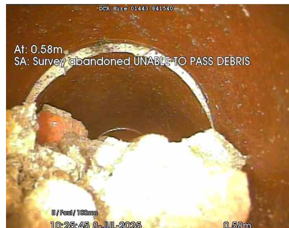
MH05 BR3_0-58m_102545.jpg, 00:00:21, 0.58 m Survey abandoned, UNABLE TO PASS DEBRIS
