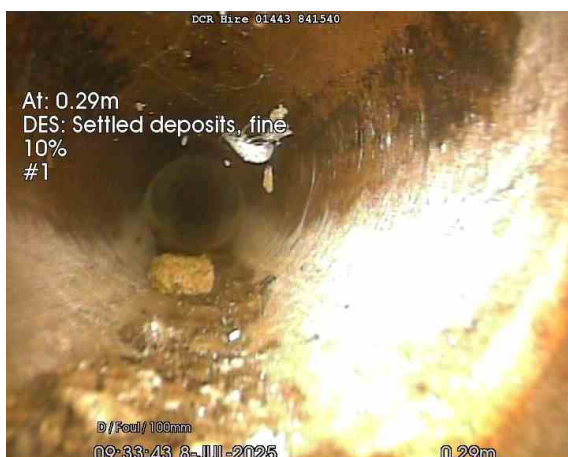
MH01 DS_0-29m_093343.jpg, 00:00:04, 0.29 m Settled deposits, fine, 10% cross-sectional area loss, start
