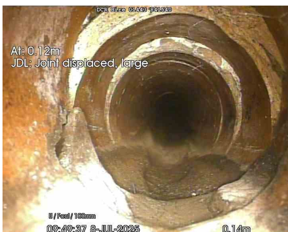
MH03 US_0-14m_094937.jpg, 00:00:08, 0.14 m Joint displaced, large
