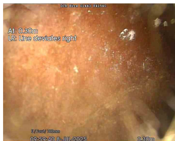
MH03 BR4_0-30m_095940.jpg, 00:00:13, 0.30 m Line deviates right
