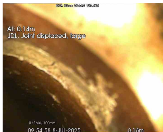
MH03 BR2_0-16m_095458.jpg, 00:00:16, 0.16 m Joint displaced, large
