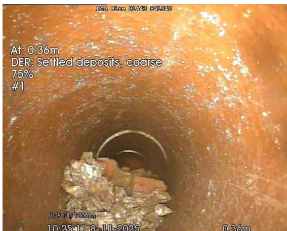
MH05 BR3_0-36m_102511.jpg, 00:00:10, 0.36 m Settled deposits, coarse, 75% cross-sectional area loss, start
