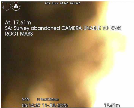
FW2301 US_17-61m_061427.jpg, 00:02:00, 17.61 m Survey abandoned, CAMERA UNABLE TO PASS ROOT MASS
