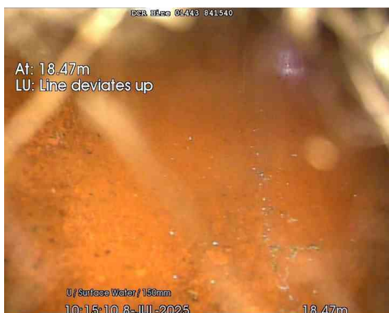
MH04 US_18-47m_101510.jpg, 00:01:07, 18.47 m Line deviates up
