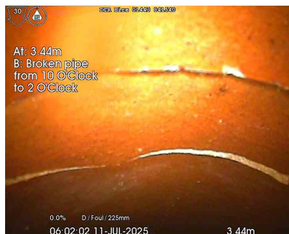
FW2301 DS_3-44m_060202.jpg, 00:00:47, 3.44 m Broken pipe from 10 o'clock to 2 o'clock
