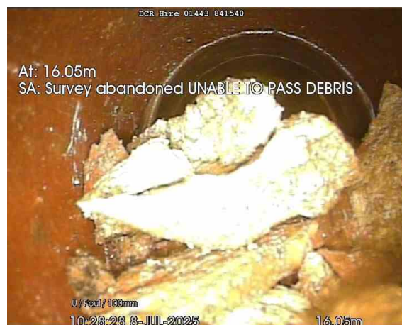
MH05 US_16-05m_102828.jpg, 00:01:01, 16.05 m Survey abandoned, UNABLE TO PASS DEBRIS
