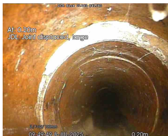
MH03 US_0-20m_094949.jpg, 00:00:13, 0.20 m Joint displaced, large
