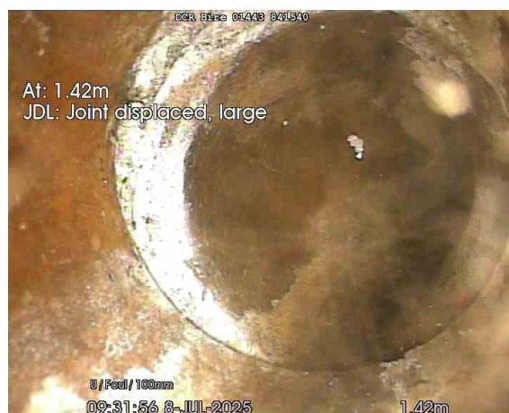
MH01 BR1_1-42m_093156.jpg, 00:00:11, 1.42 m Joint displaced, large
