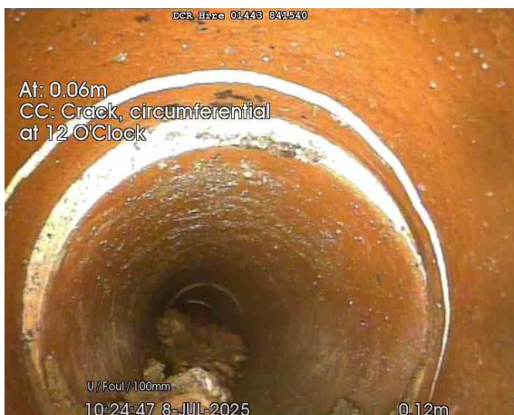
MH05 BR3_0-16m_102447.jpg, 00:00:04, 0.16 m Crack, circumferential at 12 o'clock
