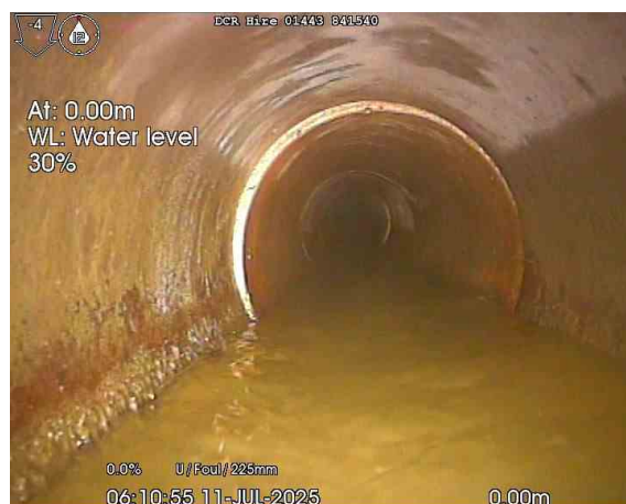
FW2301 US_0-00m_061055.jpg, 00:00:02, 0.00 m Water level, 30% of the vertical dimension
