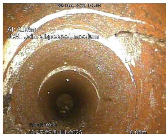
MH06 BR4_0-08m_114729.jpg, 00:00:07, 0.08 m Joint displaced, medium
