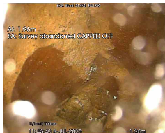
MH06 BR3_1-96m_114540.jpg, 00:00:18, 1.96 m Survey abandoned, CAPPED OFF
