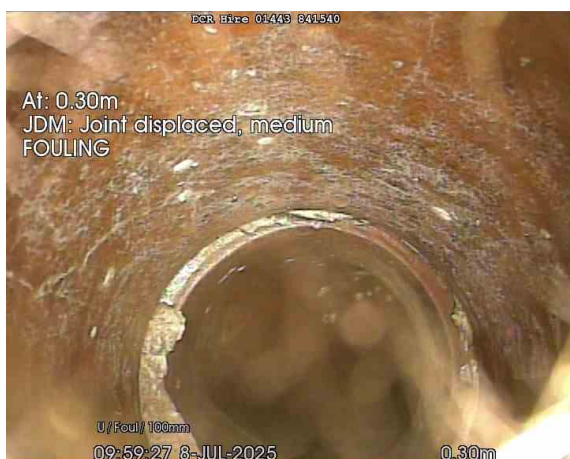
MH03 BR4_0-30m_095927.jpg, 00:00:08, 0.30 m Joint displaced, medium, FOULING
