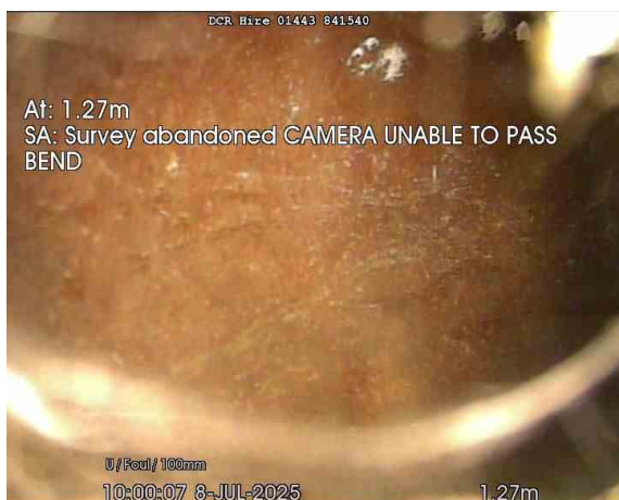
MH03 BR4_1-27m_100007.jpg, 00:00:24, 1.27 m Survey abandoned, CAMERA UNABLE TO PASS BEND
