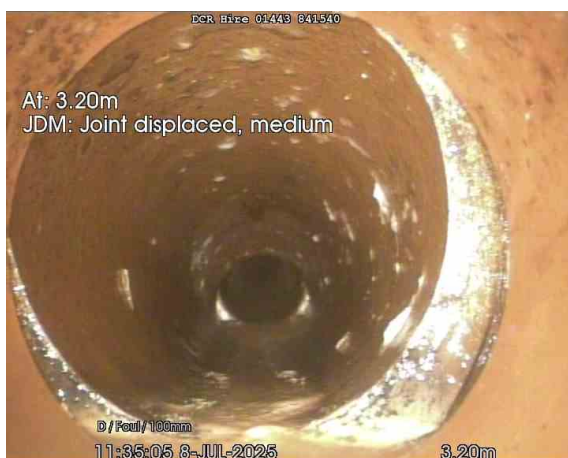
MH06 DS_3-20m_113505.jpg, 00:00:32, 3.20 m Joint displaced, medium
