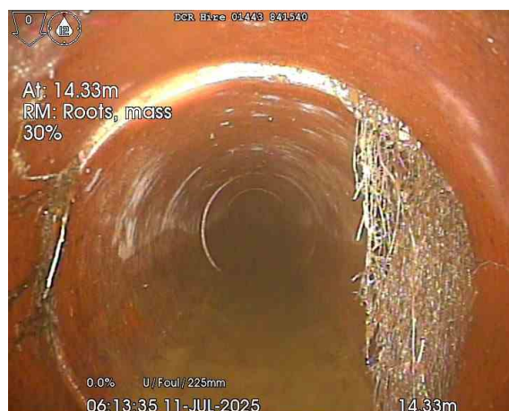
FW2301 US_14-33m_061335.jpg, 00:01:39, 14.33 m Roots, mass, 30% cross-sectional area loss
