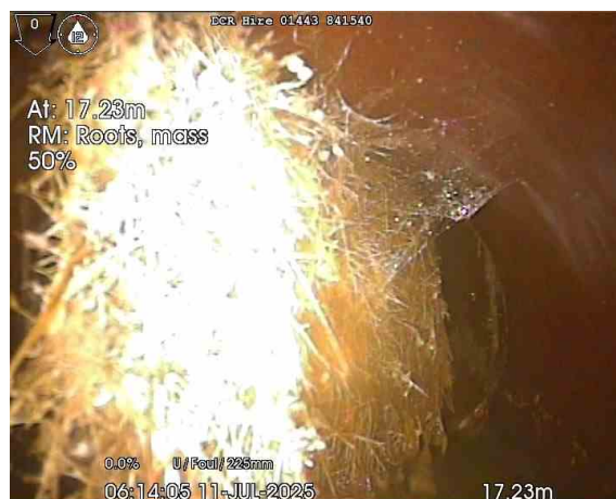
FW2301 US_17-23m_061405.jpg, 00:01:55, 17.23 m Roots, mass, 50% cross-sectional area loss
