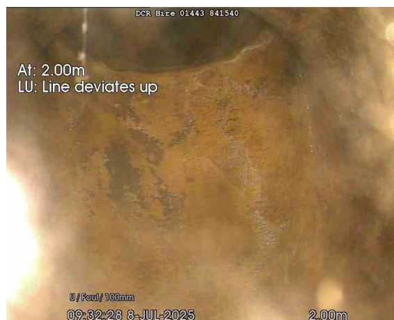
MH01 BR1_2-00m_093228.jpg, 00:00:33, 2.00 m Line deviates up
