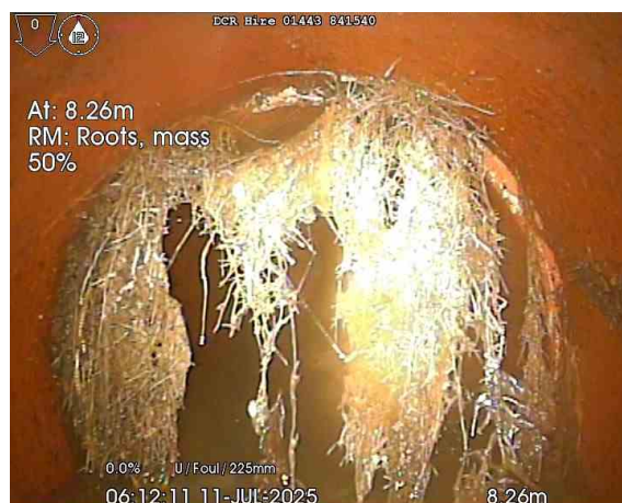
FW2301 US_8-26m_061211.jpg, 00:00:56, 8.26 m Roots, mass, 50% cross-sectional area loss
