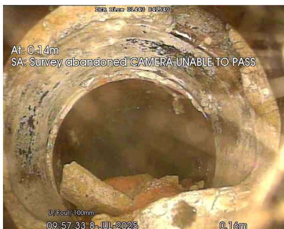
MH03 BR3_0-16m_095733.jpg, 00:00:35, 0.16 m Survey abandoned, CAMERA UNABLE TO PASS
