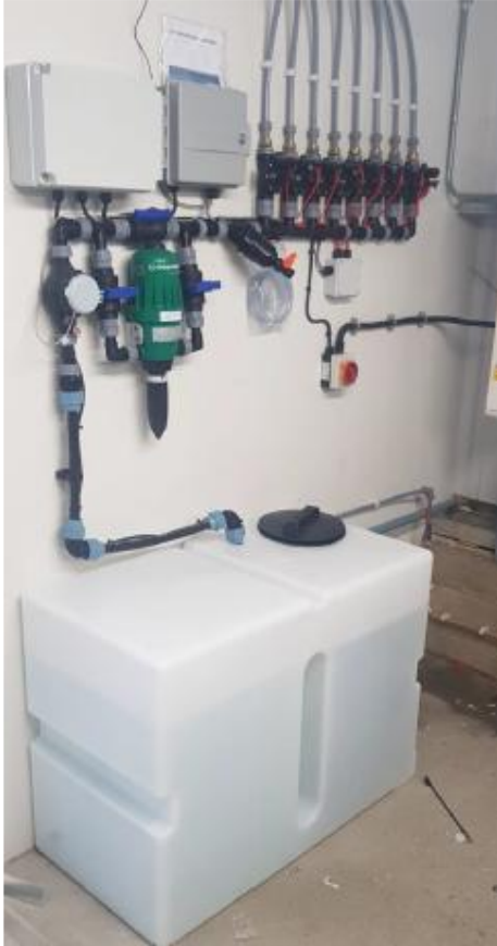
In situ, with water tank
