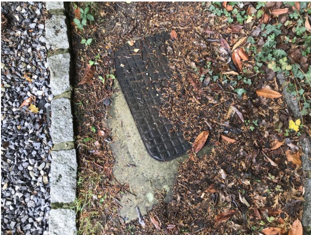
Photo 15 - Inspection chamber FRC
