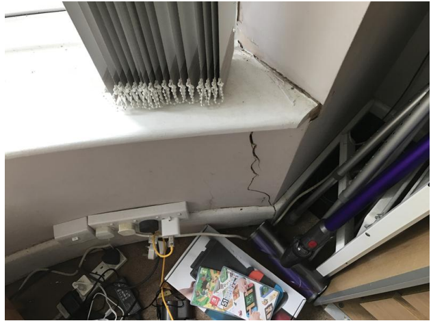
Photo 28 - Tapering crack LHs of bay window
