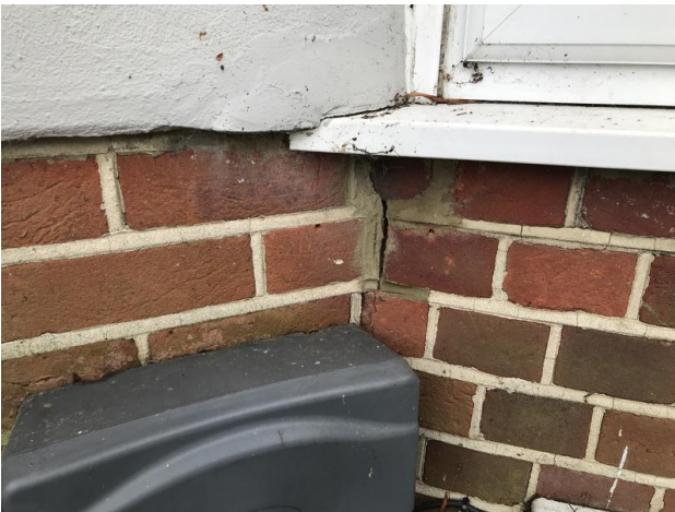
Photo 20 - Open joint at junction with front elevation
