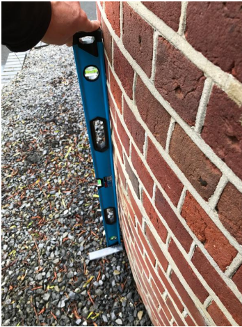
Photo 22 - Slight tilt and rotation of dado wall
