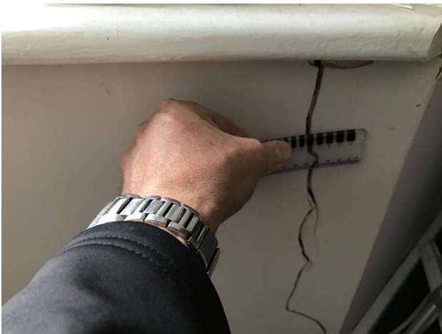
Photo 29 - Crack width 5 mm
