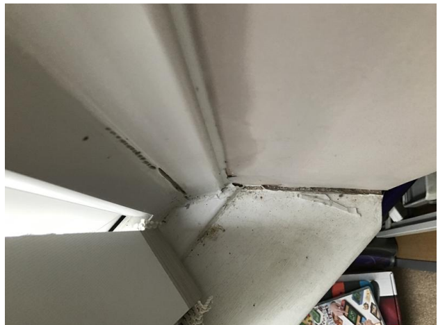
Photo 30 - Distortion continues into window frame
