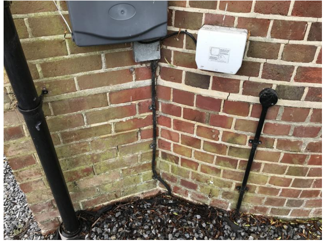
Photo 19 - Cracking LHS of front bay window
