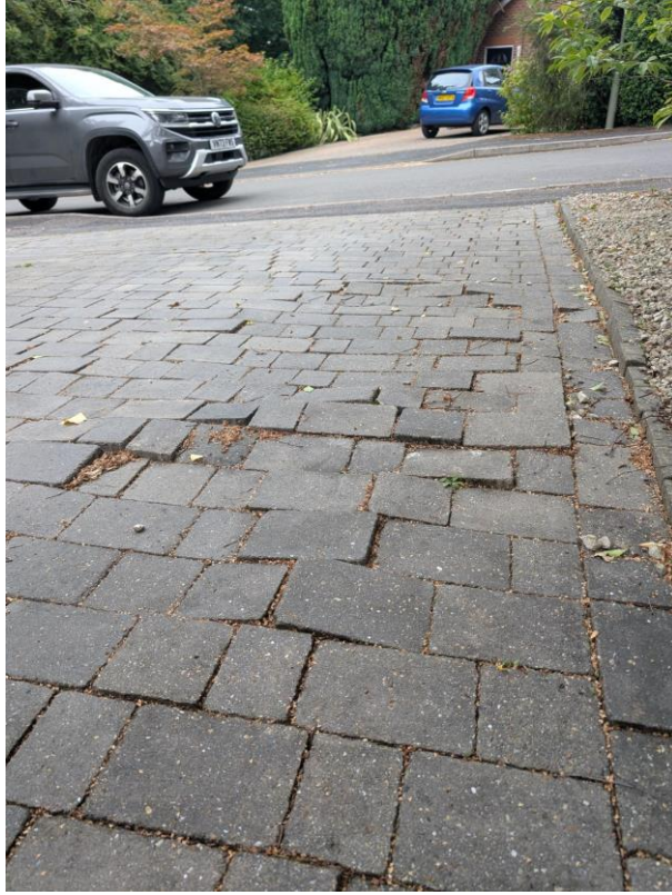
T1 – Driveway immediately adjacent to T1 displaying raised and uneven paving stones.
