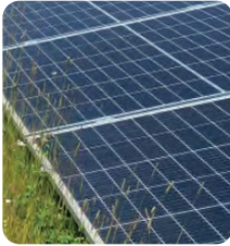
Photovoltaic Roof Panels
