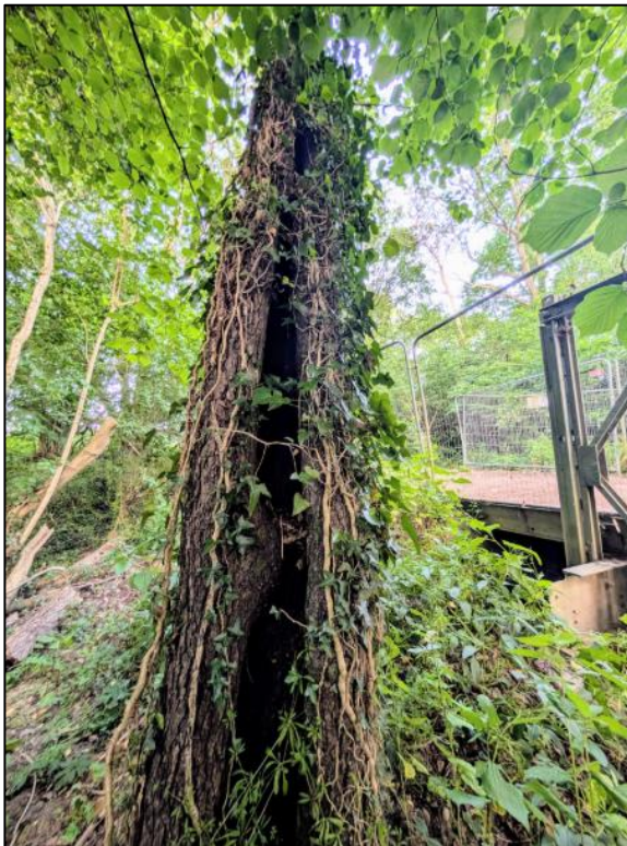
Photo 11 Tree 1 – Large trunk cavity that runs halfway up the tree
