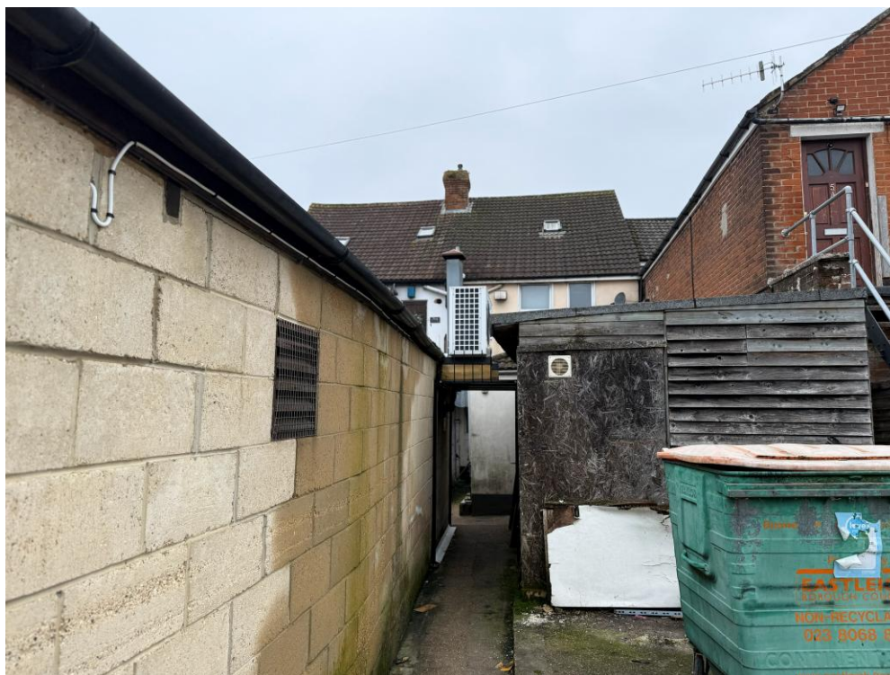
Figure 6 – Condensing Units located above the existing covered walkway.
