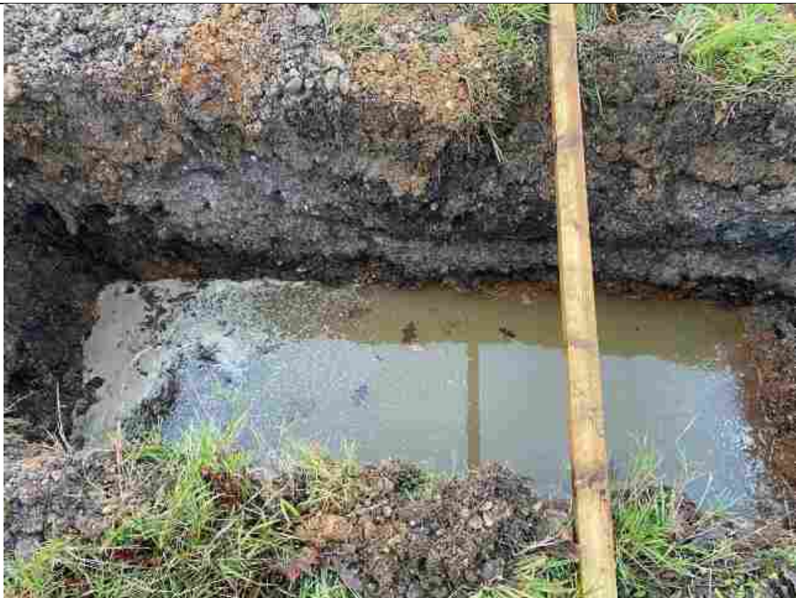
PLATE 21 – Standing water level in Structure 5 trial pit the following morning
