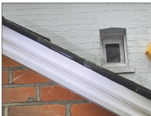
Figure 5 – Gaps present between the barge boards and slate roof tiles.
